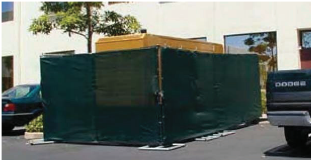
Figure 5-26 Example of Inappropriate Ground Mounted Equipment Screening
