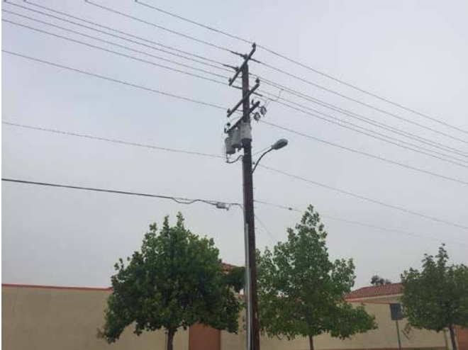
View of a pole mounted transformer on the adjacent property to the west
