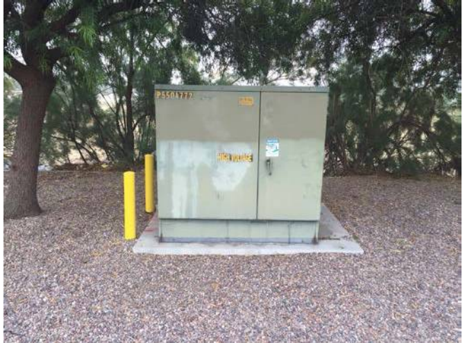
View of slab mounted transformer on the adjoining property to the west
