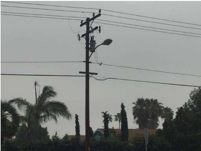
View of a pole mounted transformer on the adjacent property to the north
