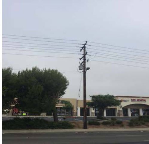
View of a pole mounted transformer on the adjacent property to the west
