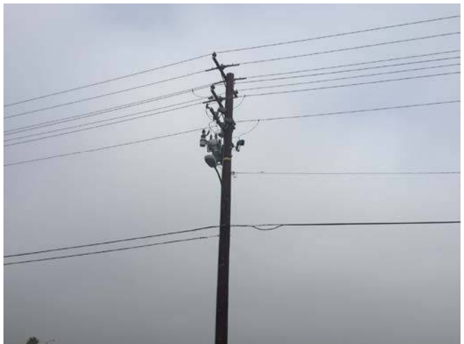
View of a pole mounted transformer on the adjacent property to the west
