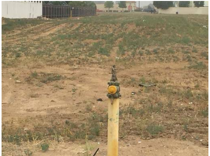
View of municipal water on the Property
