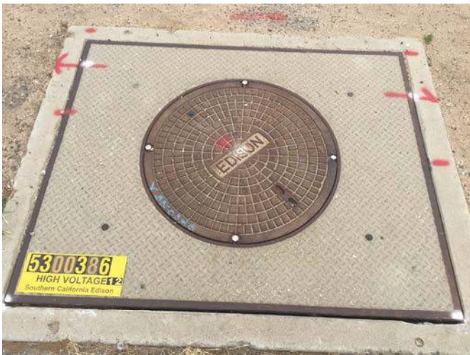
View of an underground transformer on the Property on the south side
